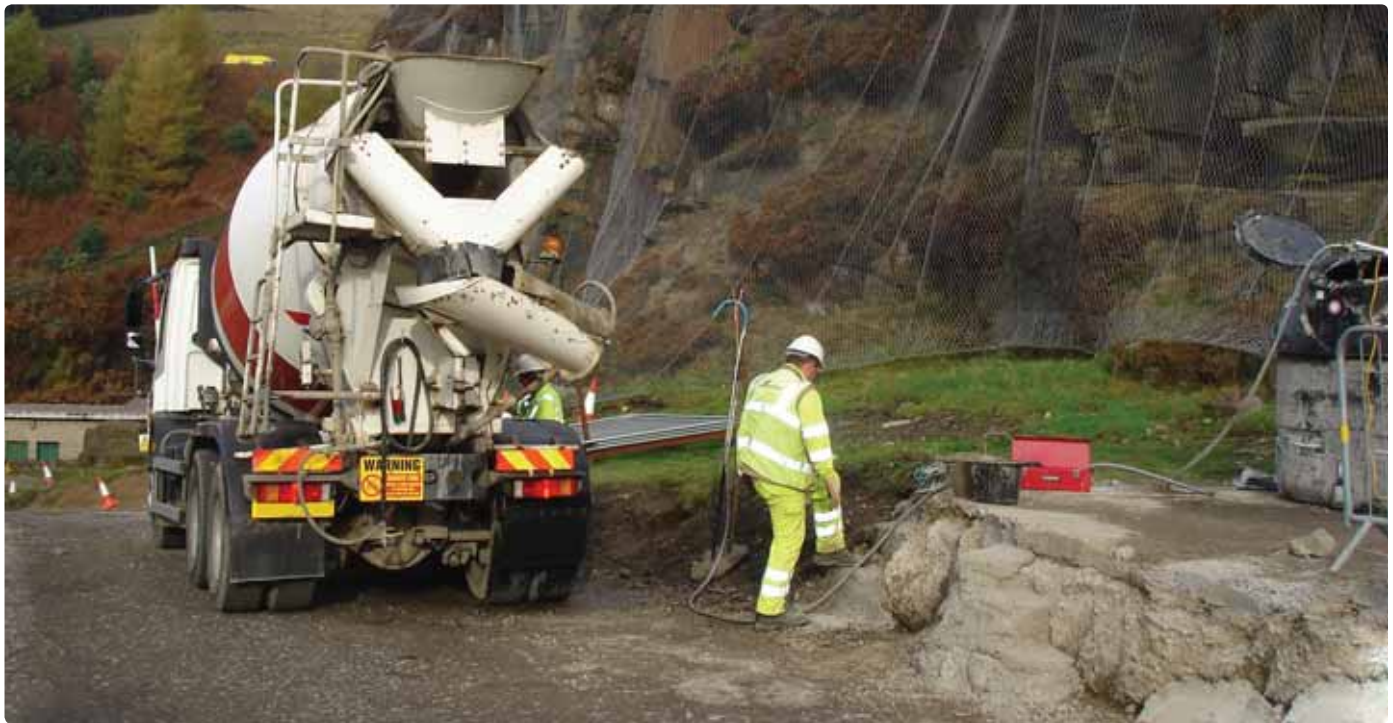
Figure 3 above: Addition of superplasticiser to the concrete immediately before entering the tunnel from the western end.
