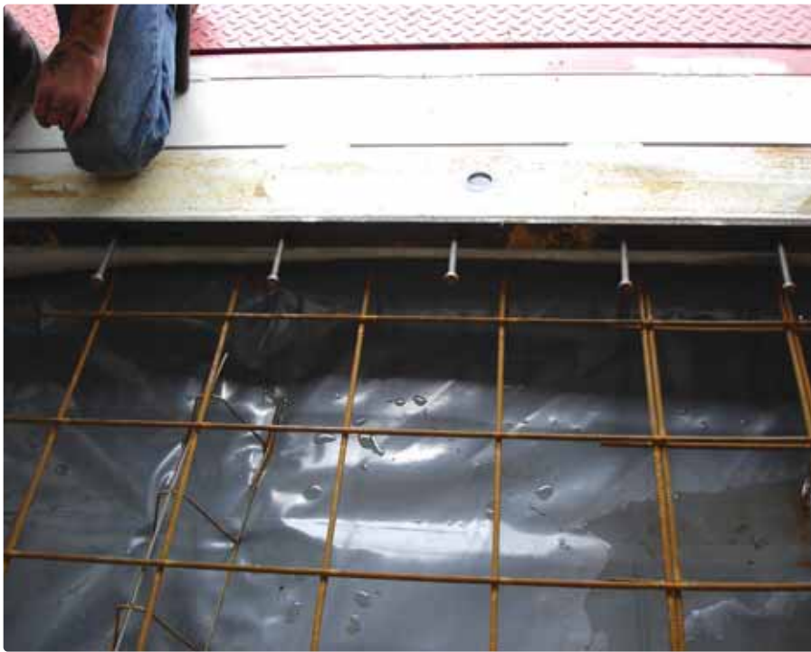
Figure 6 above: As Figure 5 with Strip Joint ready to be cast into the floor edge.
