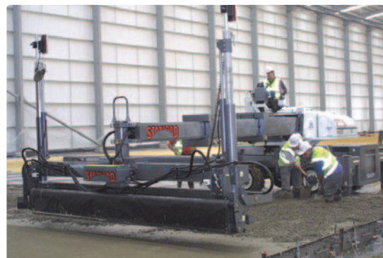
Figure 2: Current specifications call for a precision approach to all aspects of floor installation, including formwork, laser-screeding and dry-shake application.
