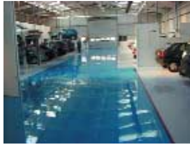
Figure 3: This pigmented floor exhibited excellent abrasion resistance and was used in a vehicle servicing area.
