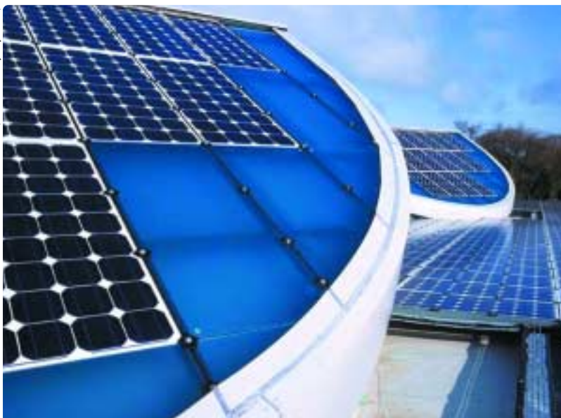
Figure 1: Directional photovoltaic cells on the roof of Chulmleigh School.
